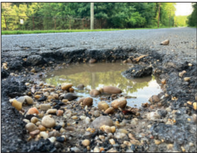
This hole's depth is disguised by the water in it. Woe the cyclist who encounters it.
