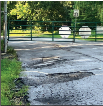
The gate to BARC is warded by a series of potholes and a speed bump.
