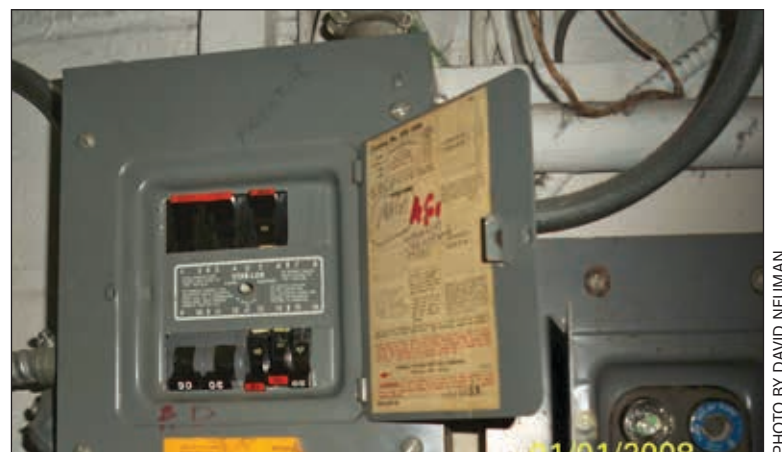
Stab-lok panels, manufactured primarily by Federal Pacific (FPE) or Federal Electric (FEP), remain in various buildings and complexes around Greenbelt. Even where installed legally, their circuit breakers are unreliable in preventing fires. With either Stab-loks or overfusing, it is especially critical to monitor what we plug in, because an overload may not be automatically interrupted in time to prevent a fire.
