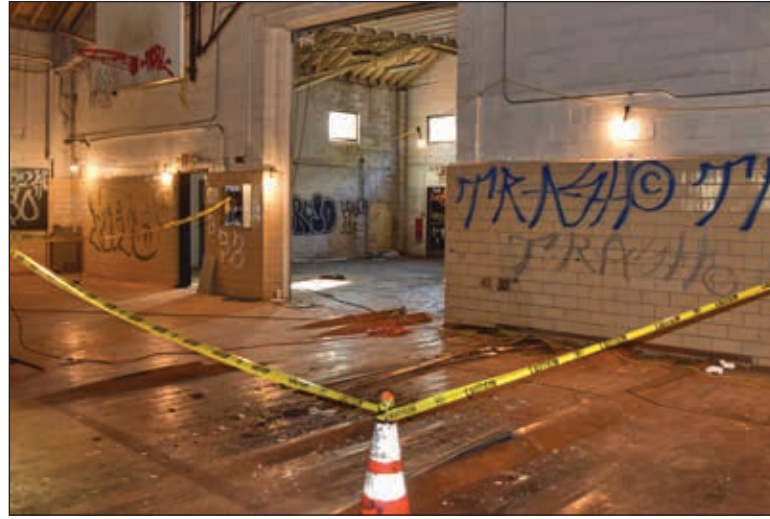
A damaged roof has led to water damage that impacts the ceilings and floors of the Armory.
