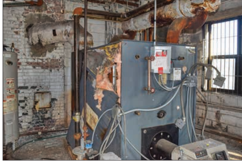
The Armory's boiler room at the time of acquisition
