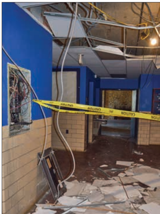
When council toured the Armory building in October, following the acquisition, they found that copper wires had been stripped from electrical boxes, the ceiling bowed and rubble filled the corridor.
