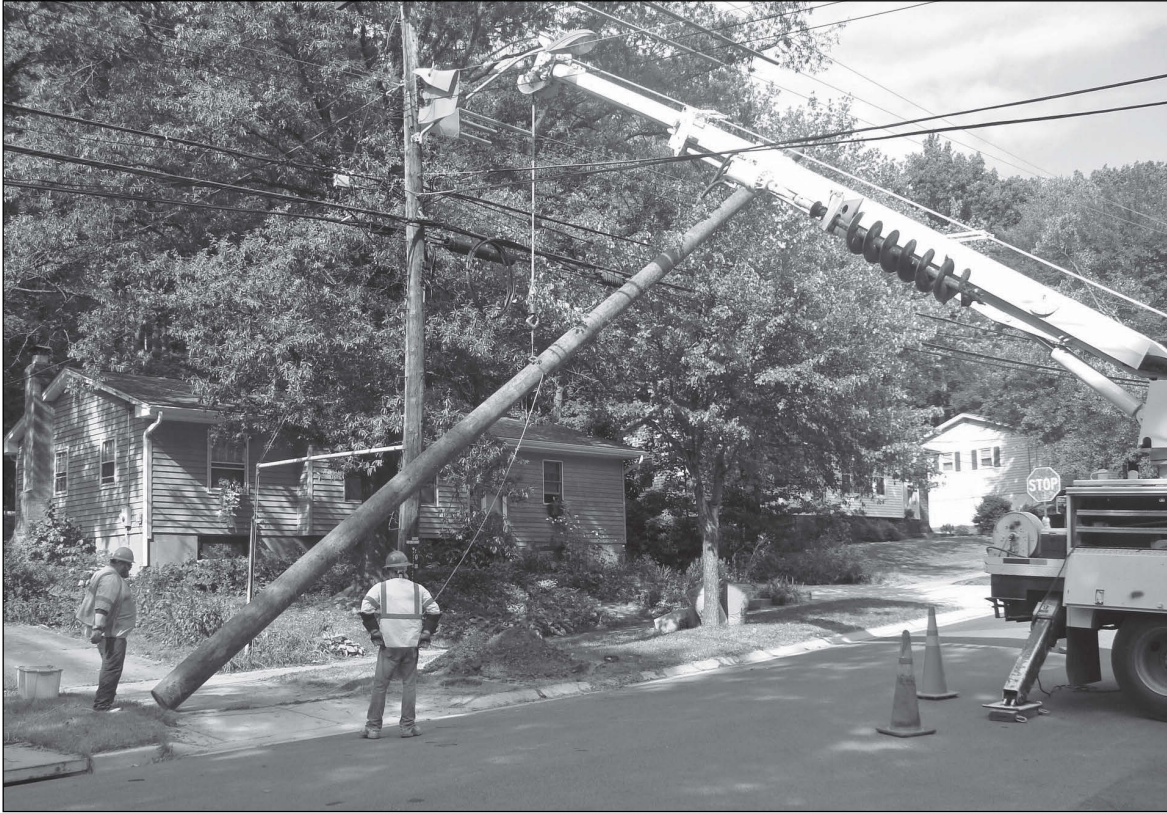
John Gochnour (left) and Brian Marmo watch as the new pole is raised. When it is perpendicular and the butt end rises off the ground, they will guide the size 2 pole into the 7 ft. deep hole. The next steps are to plumb the pole, backfill the hole and tamp using a pneumatic device.
