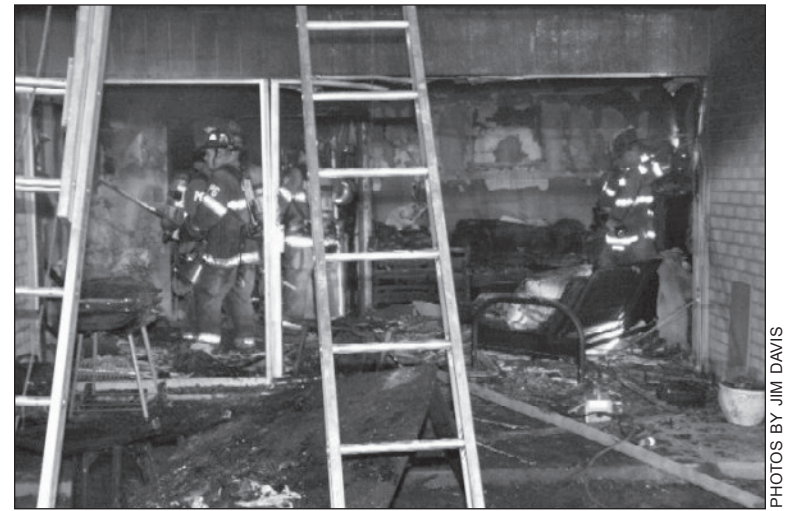
Burned out ground level apartment.
