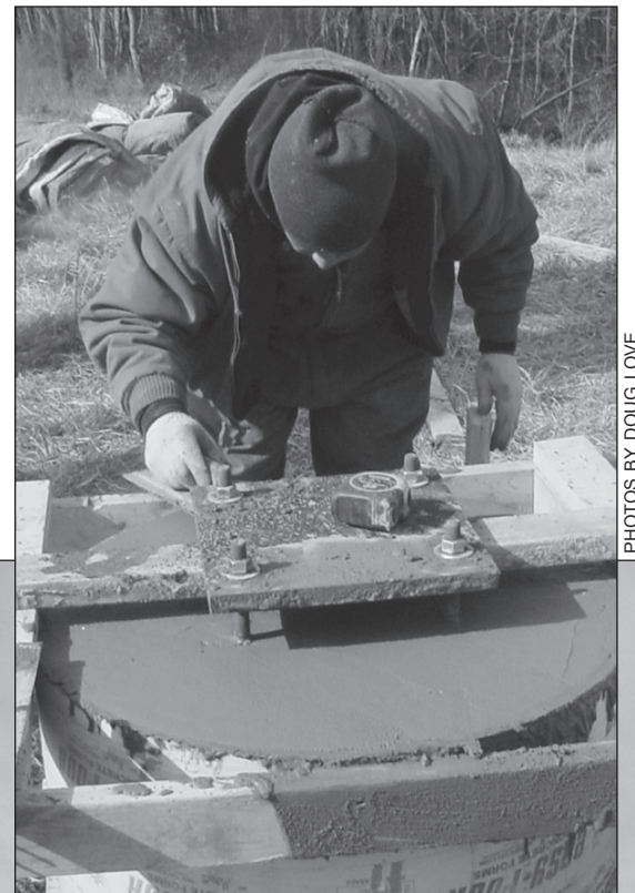
At right, Herman finishes trowelling the top of the pier with the bolts in place for the observatory. After all the work is done Doug Love dates the wet concrete. The pier was then covered with warming blankets to protect against the coming snow and ice.
