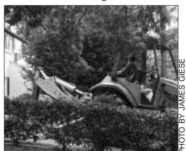
Prospective contractors worked to provide a way to save this large American holly tree at 62 Crescent Road. The award was made to a company that will tunnel under the tree to replace damaged pipes.
