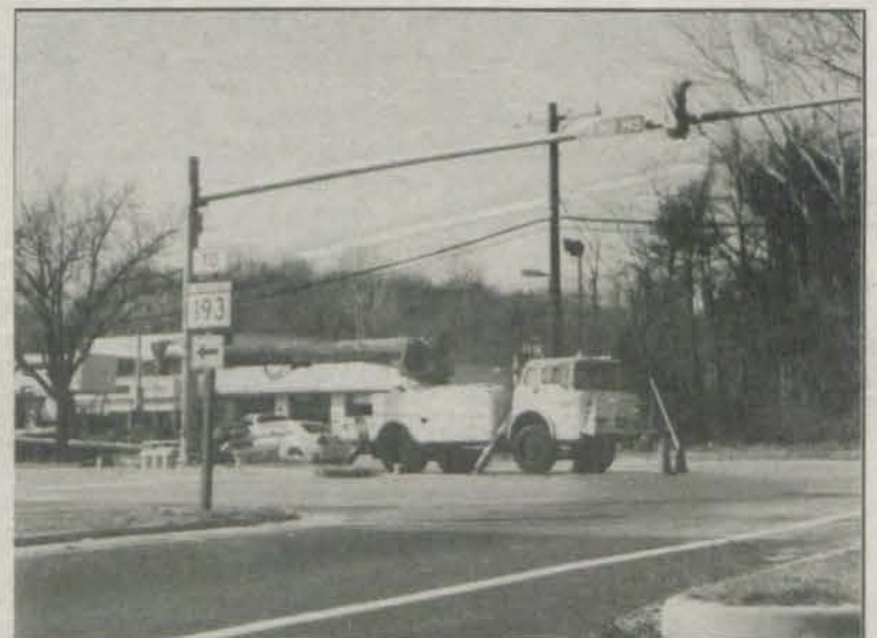
Newly installed traffic light on Southway will be activated soon.
