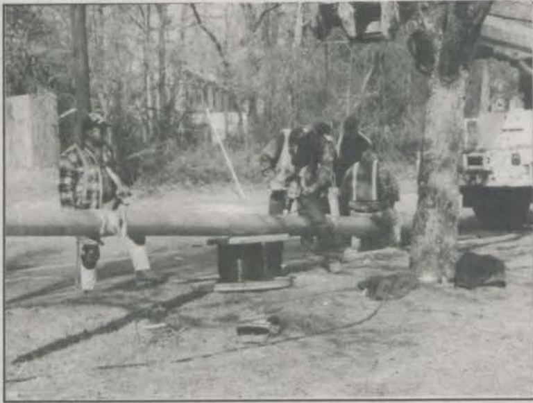
Workers install a new traffic light on Southway near the Citgo station. - photo by Judy Nelson
