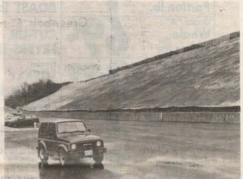
The East Slope adjacent to Beltway Plaza was restabilized and planted in the Fall of 1992.
