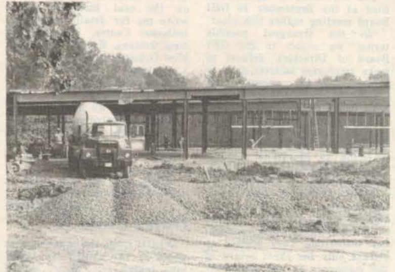
Concrete flooring and steel framing are being installed as the new elementary school on Ridge Road begins to take form. —photo by J Henson
