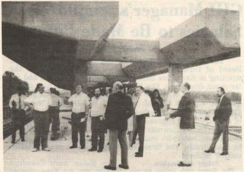
METRO officials explain layout of the Greenbelt E Route station and parking lot to Greenbelt officials during a tour of the station now under construction and to be completed next year. —photo by Ray McCawley
