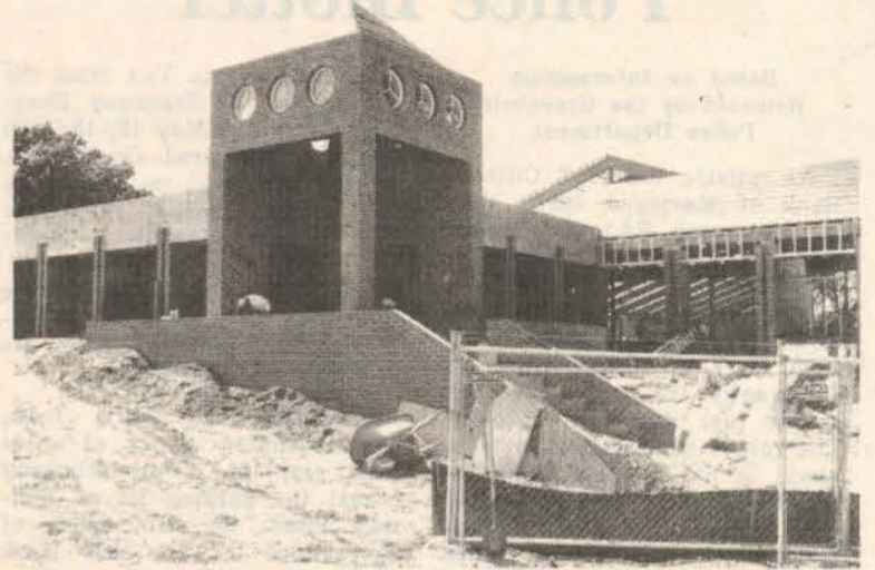
The main entrance of the indoor pool, under construction here, features porthole windows that tie into the design of the outdoor pool building. — photo by J. Henson
