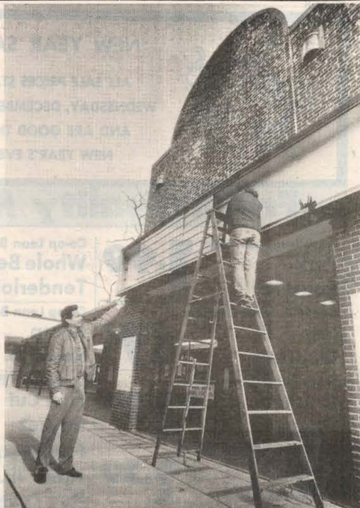
Paul Sanchez talks with workman repairing the old marquee. — photo by J. Henson
