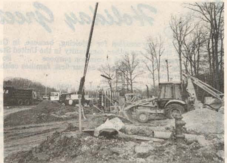
Crane, bulldozers, dump trucks at work on the indoor swimming pool site. — photo by J. Henson
