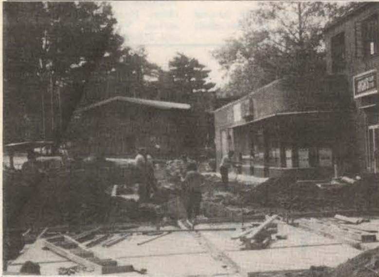
The west end of Centerway is cleared and regraded in preparation for a new sidewalk, curb and gutter and landscaping. — photo by Diane Oberg
