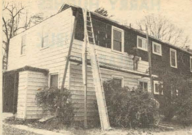
The final dressing! Siding the GHI frame homes is now well underway. The entire job is expected to take a year.
