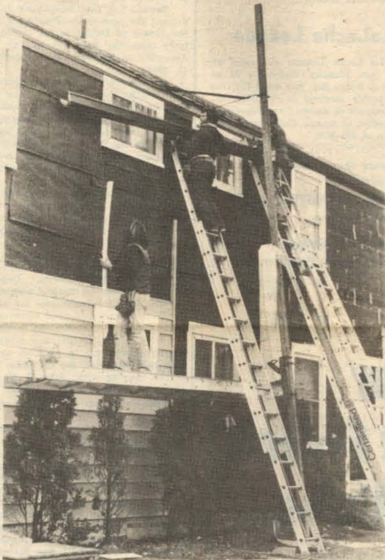
With the aid of ladders and scaffolding, teams of workers from Beltway Aluminum install vinyl siding from Research to Southway in a variety of colors.
