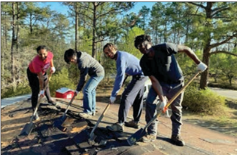
Members of MCF Community Church work on a roof for a house in need of repairs.
