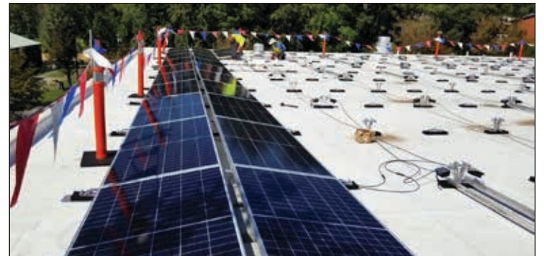
A pristine roof and solar. What more can a Co-op's heart desire?
