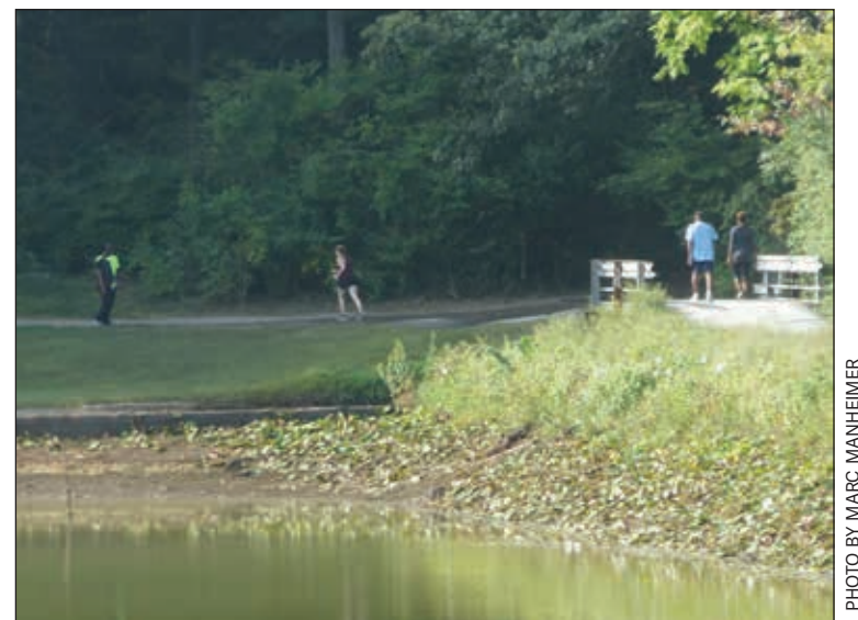
The water level at Greenbelt Lake is visibly low as construction begins on the dam. The path along the dam will remain open for the next few months while work proceeds on the downhill side of the dam.
