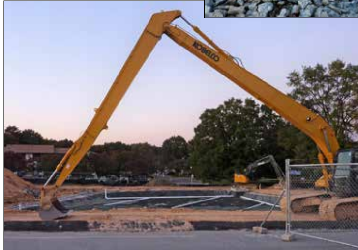
Construction of a filtration system at ERHS will help keep pollutants out of the storm water systems.
